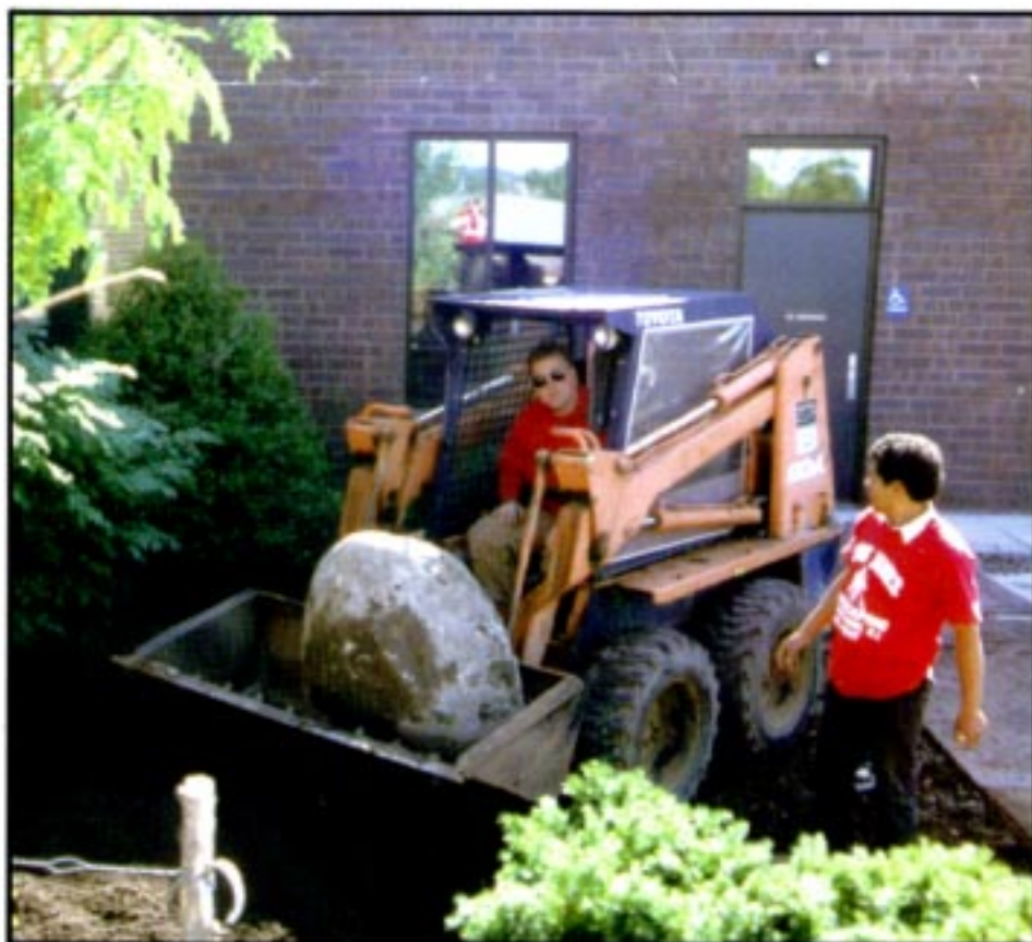
(L-R) Chris James and Omar Ramos are doing a landscape installation at Robertet Inc. in Oakland, NJ.
